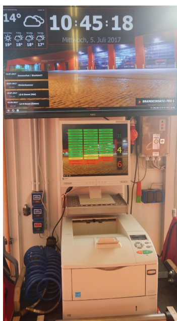
Picture 29: Complex alarm system for a voluntary fire station without personal attendance in Lübeck, Germany
