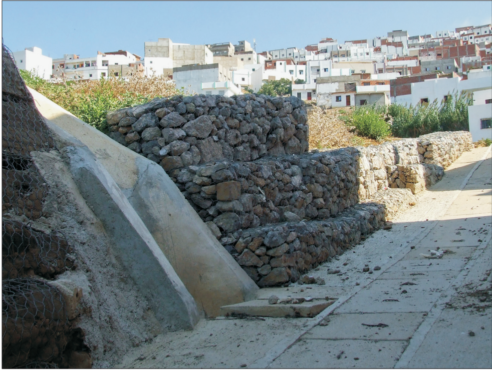
Photo 3. Protective wall between the road and the slope after landscaping (10 x 10 m). (Photo by Prokos, H. 2013)
